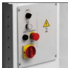
Panel de control
